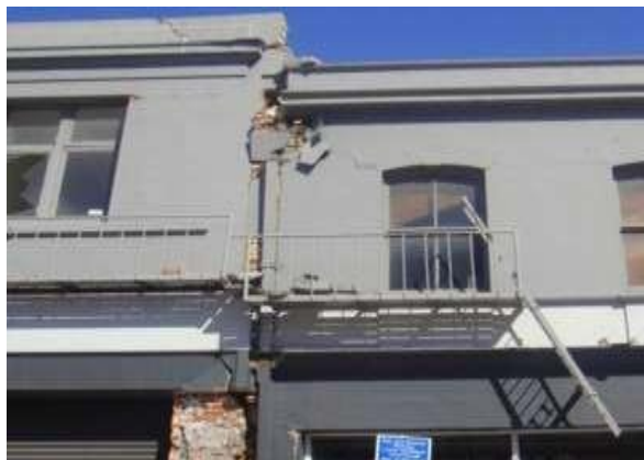
Fig. 1. Pounding damage observed in Christchurch CBD
